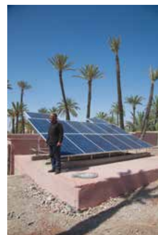
The wells were equipped with solar panels to avoid CO2 emissions.
